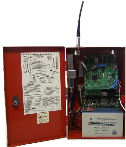
An Intellitize Subscriber Unit with MMX Installed
